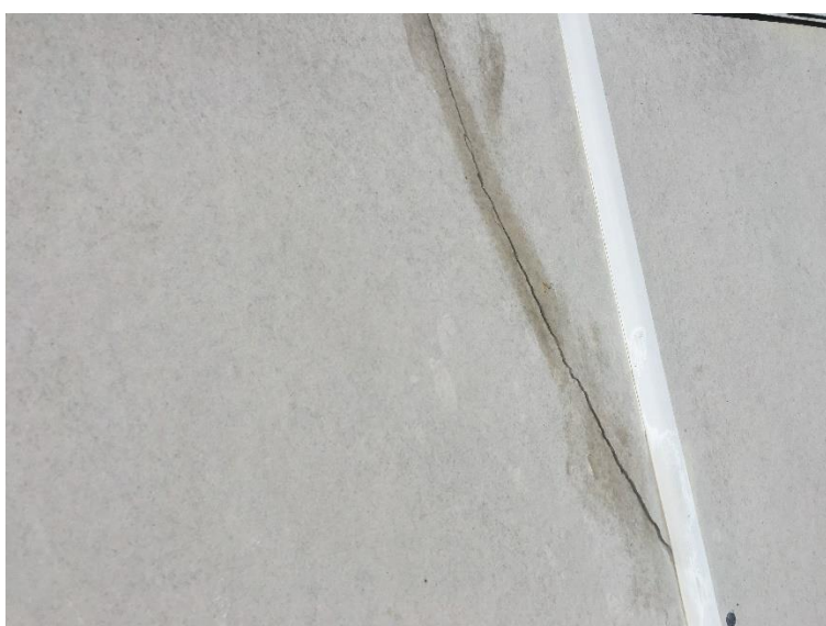
Crack through pp sheet at squash court – timber frame above concrete wall
