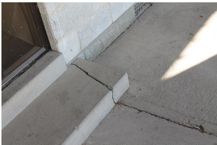
Crack through step at veranda
