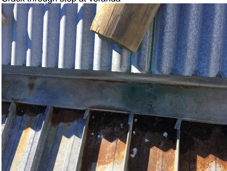
Rust on roof at box gutter
