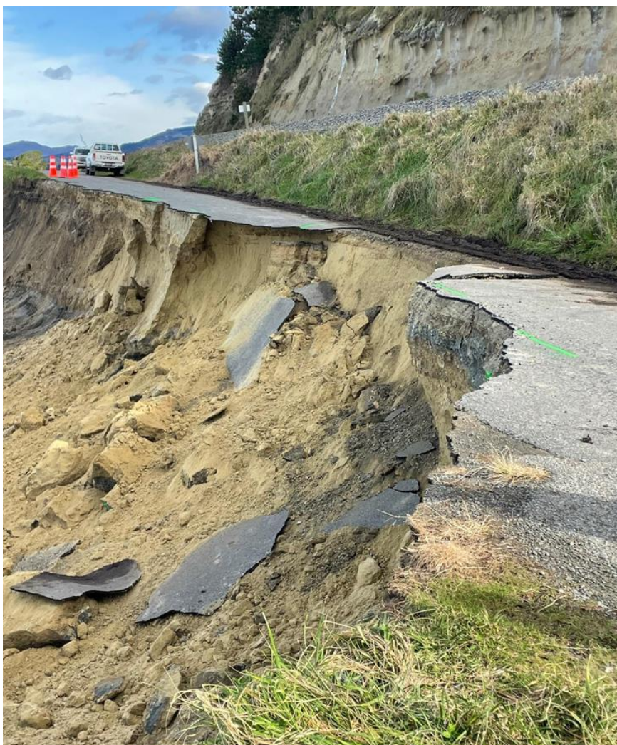
Figure 2.1: Erosion and slope failure of Claverley Road. Photo taken on 13th July 2023.
